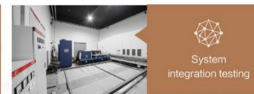
Electric control system lab
